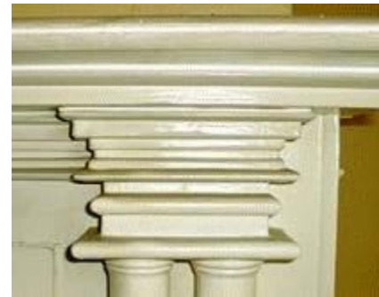
The front entrance columns and pediment, widened doorways and columns in the front hall, and first floor mantels were among the alterations made in 1905.
