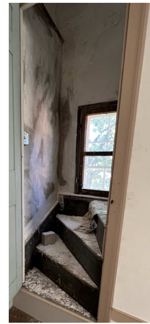
ATTIC STAIR PLASTER
